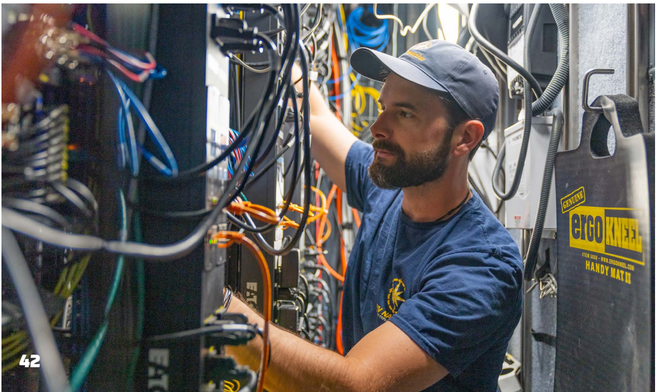
FIGURE 1. An all new fiberoptic backbone connects E/V Nautilus's rack room with the control vans and other key areas of the ship.
